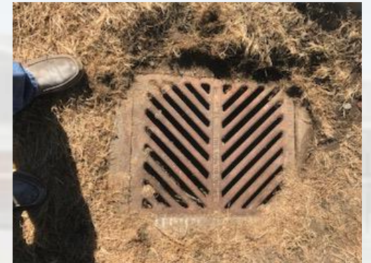
Storm drain raised 12 inches to remove Trip hazard.
