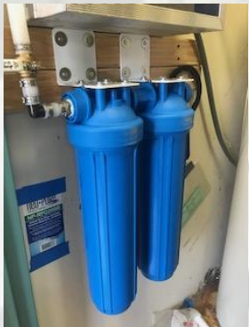
New filter assembly for drinking water At WPS
